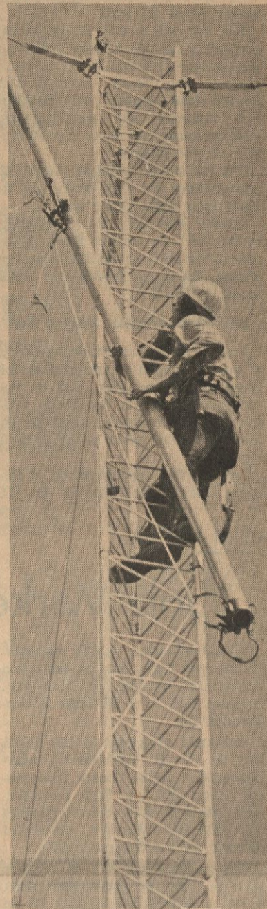
TOWER TAKES SHAPE. High above a hillside west of campus, Dennis Henderson of the North East Texas Communications, Co., adds another link to the 250 foot tower that will eventually broadcast ET radio station KETR-FM over a 50-mile radius.
