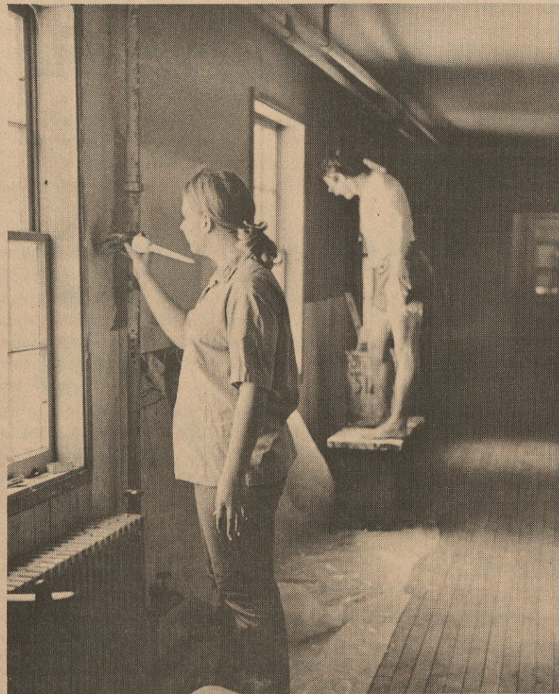
STUDENT HELP—Ree Elliff, Amarillo senior, and Garrison Ausburn, Dallas junior, are two of the students engaged in the renovation of the Speech Building. The building will be remodeled to give it an "old English barn" atmosphere.
