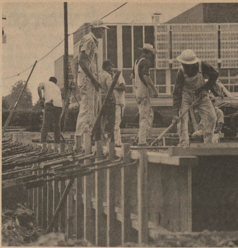
T-LOUNGE WORK —Workmen spread concrete for the foundation of the new T-Association Lounge building, which is scheduled for completion in September. The building will be located just south of Memorial Stadium and west of the Student Center. (Photo by Danny Templeton)
