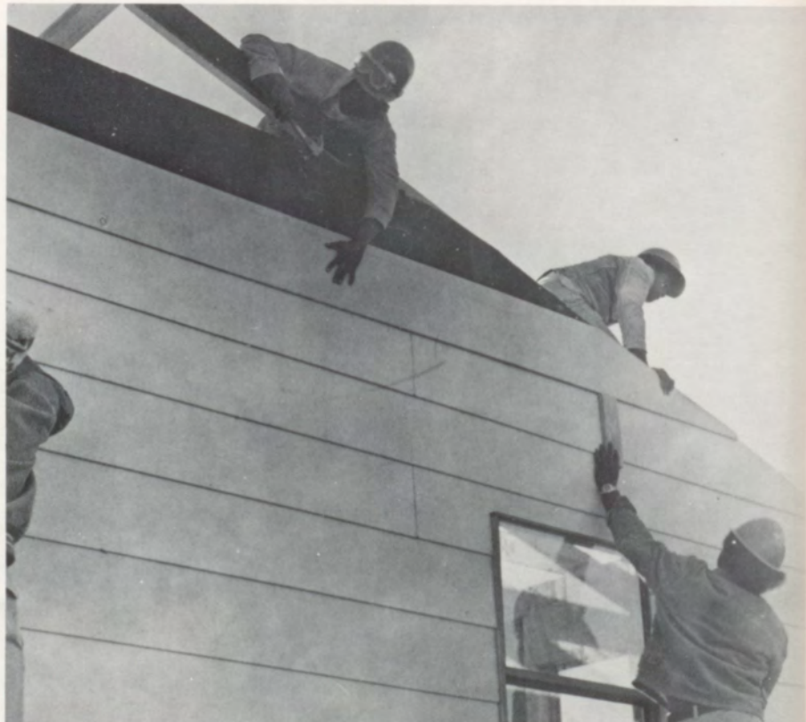
The Building Trades classes construct a house which is sold after they are finished.
